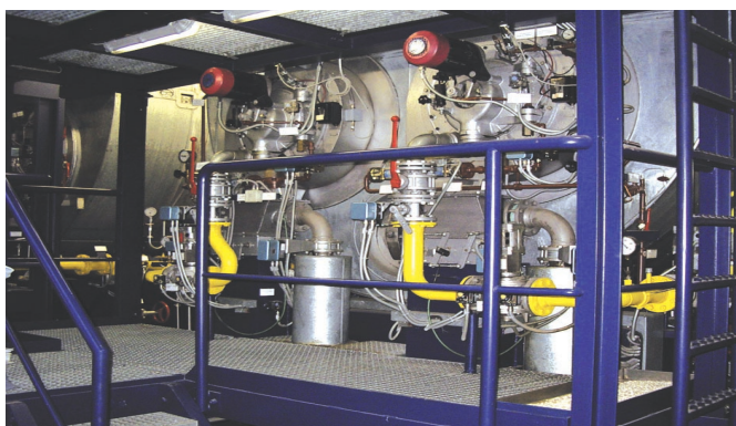
Reference installation at the Bayerische Julius-Maximilians-Universität in Würzburg: 14 MW double-fired tube hot-water boiler fitted with two Ray burners and CO regulation
